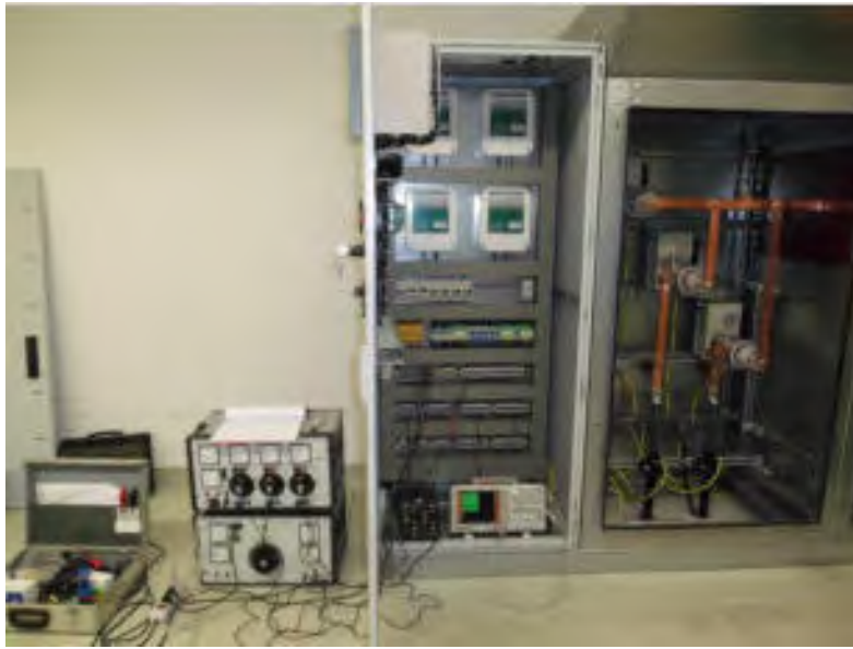
Control cabinet and switchgear panels 10.5 kV (25kA)
